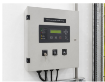
Demo control panel
