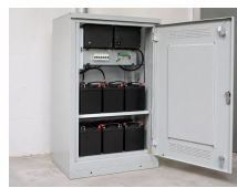
Demo battery backup
