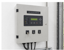
Demo control panel
